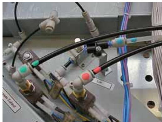
Abb. 8-8 Pipes at the nozzles
